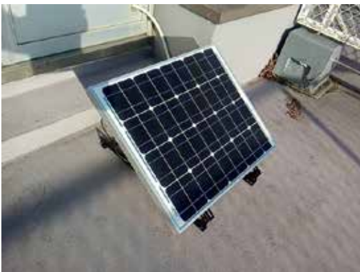
Figure 12 Installation of solar cell panel on the flat roof of the building
